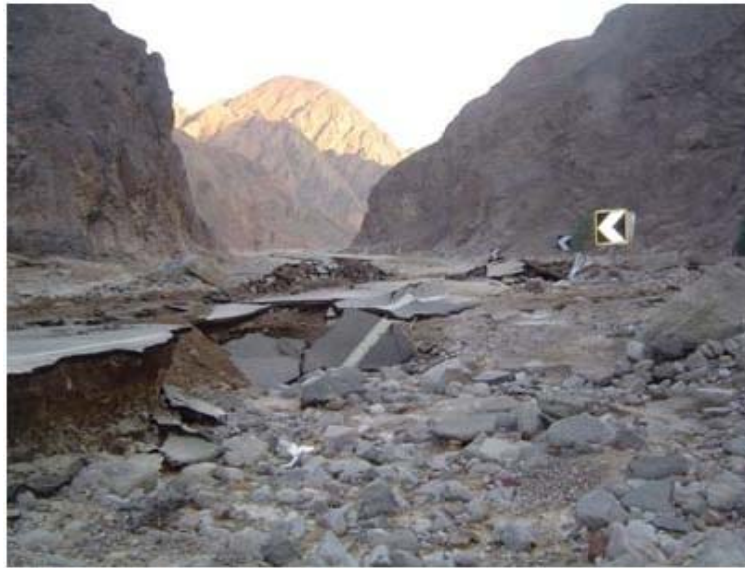
Figure 2: Severe flash flood impact on the international road
